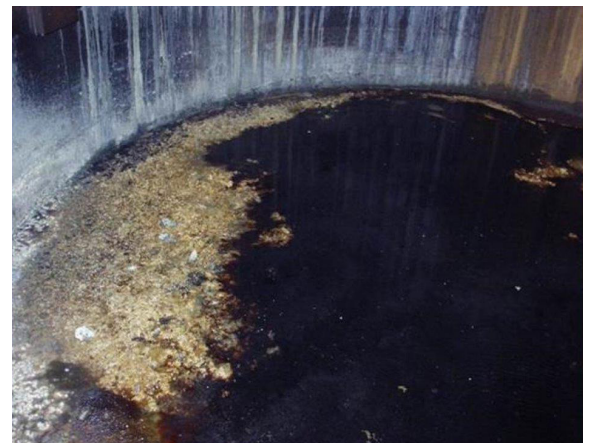
Stack Corrosion Inspection
